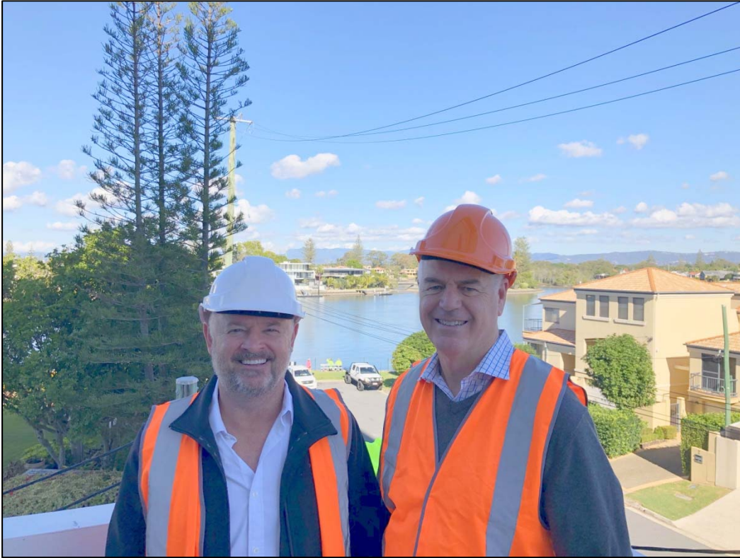
HCAP Developments CEO, Steve Howell and Marquee Development Partners CEO, Mark Spedding on site, inspecting progress at Peninsular Residences
