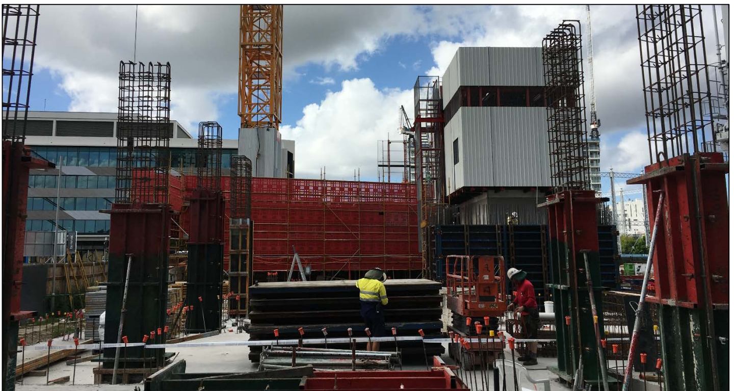
Haven Site: Formwork for columns to support the Level 1 floor slab. The white lift core jump-form is visible in the top right of the image.
