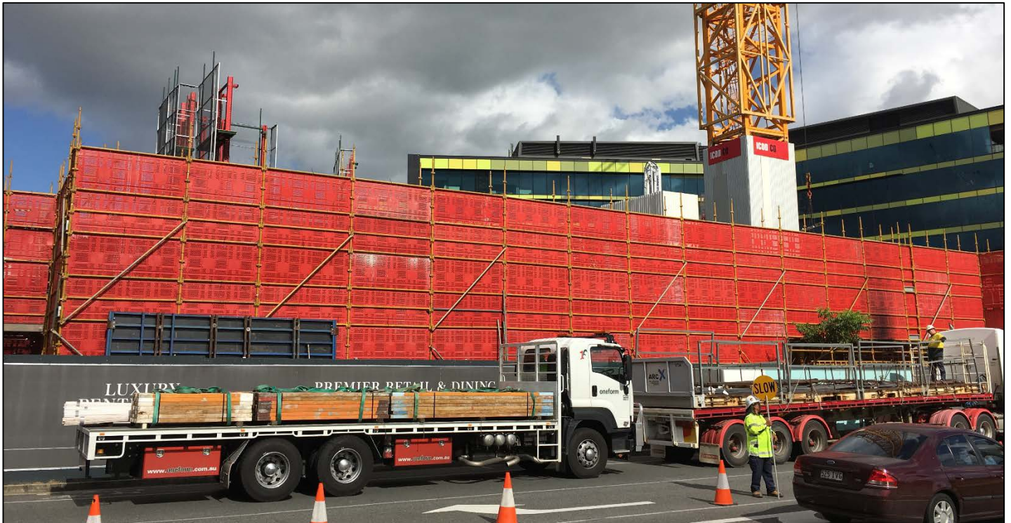
Haven Site: View from Cunningham Street showing scaffolding erected around southern portion of the tower.
