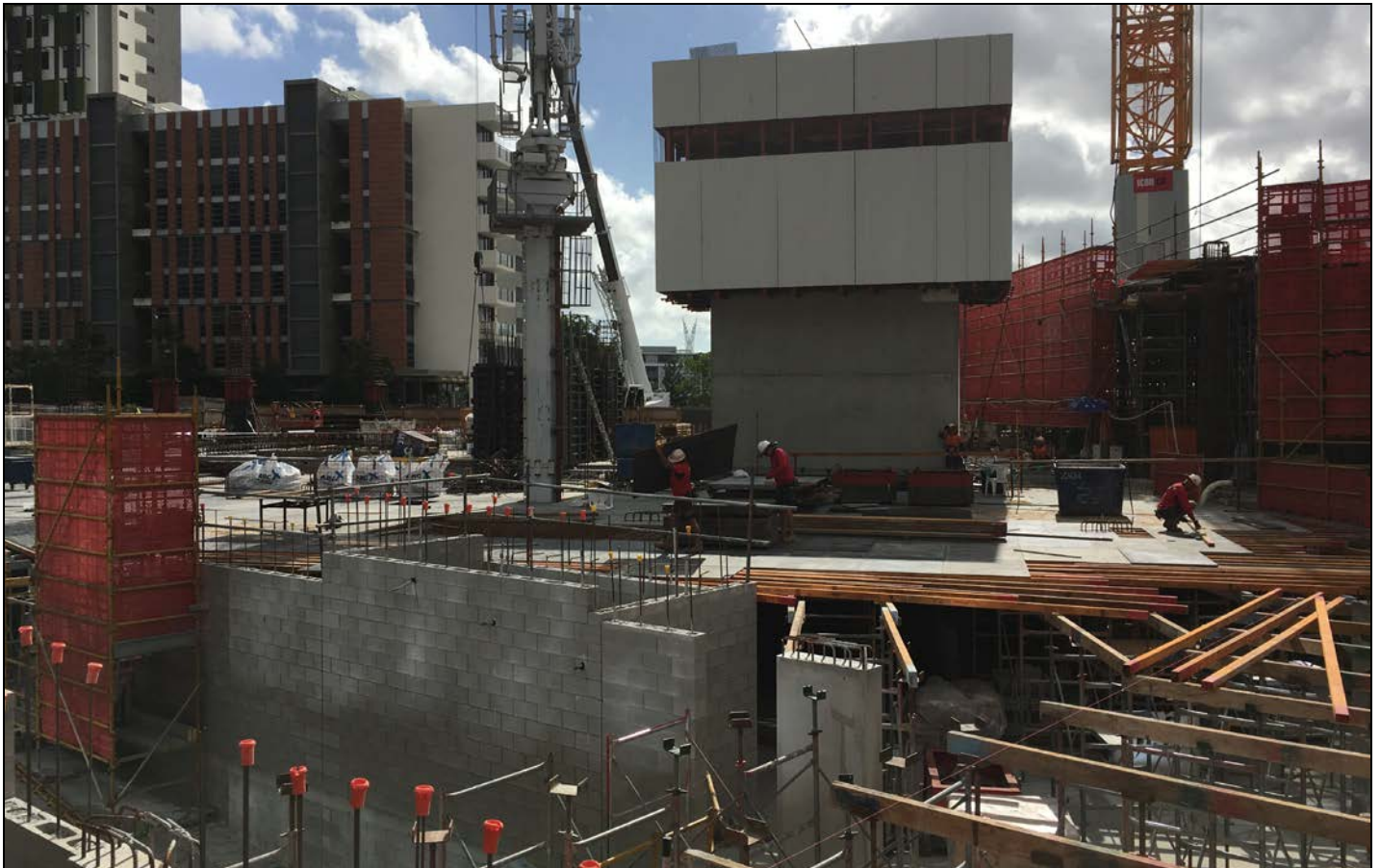
Haven Site: Haven ground level showing the car par ramp (bottom left), form-work for remaining ground floor slab (bottom right), lift core and jump-form (center), and tower scaffolding (top right).
