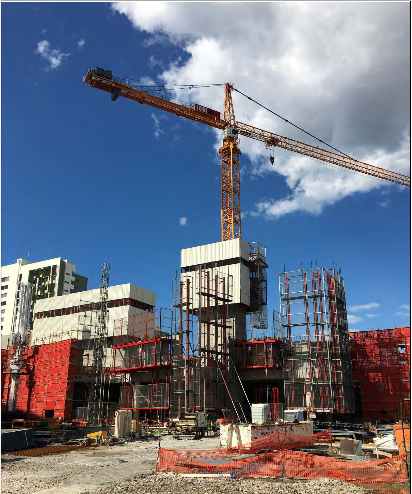
Haven Site: Easterly view of the Haven tower. The tower includes two jump-forms that will lead the construction progress up to Level 25.
