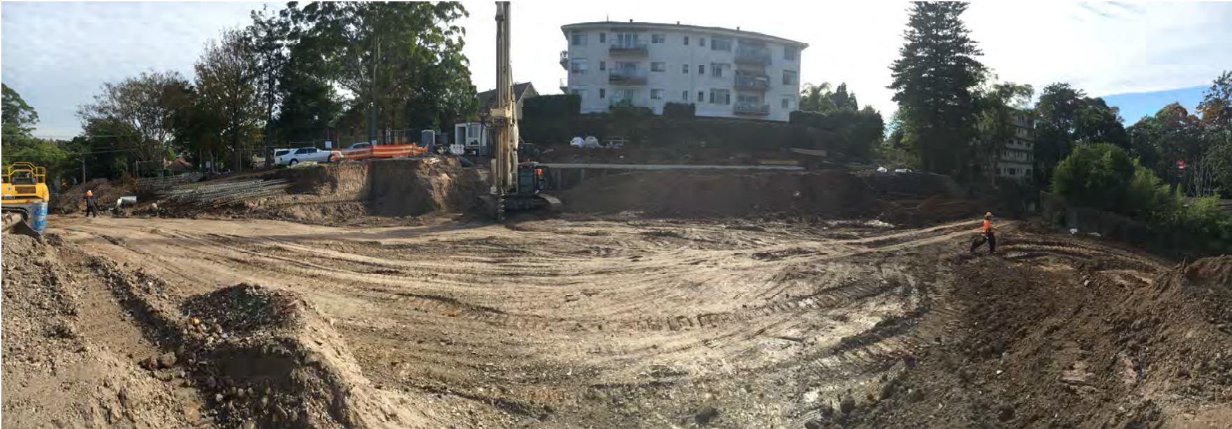
Photo 3 – The panoramas below show the site on the 29 th of April with excavators commencing the bulk out adjacent to North boundary piles.
